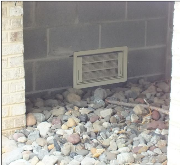
Photo 15: Flood vents installed on an elevated home.
