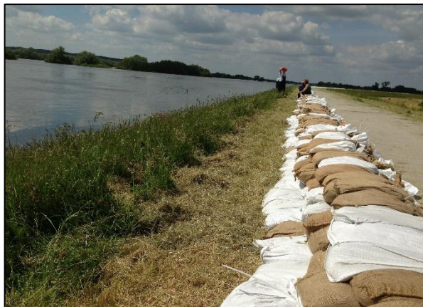
Photo 9: Sample of temporary sandbag barrier.
